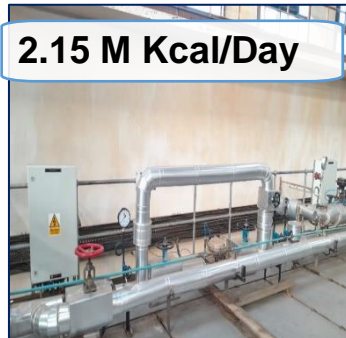
Pressure Reducing Station
