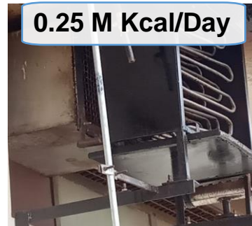
Waste Heat Recovery
